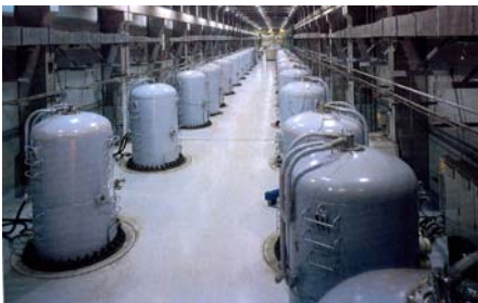
Polysilicon Deposition Chambers at REC Factory
